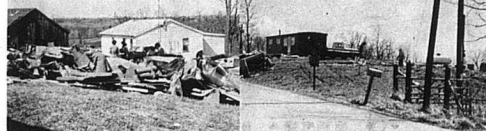
All that remains of the Helen F. Alexander trailer on Ky. 24 a short distance from Carlisle. The residents were away from home as the storm demolished their trailer.—Mercury photo
