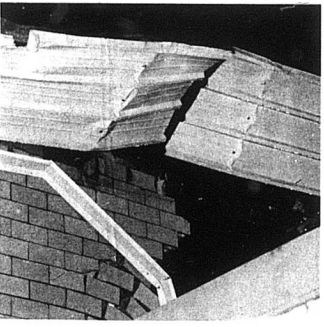
Large hole is visible as roof and wall damage at BGK Knitting.—Mercury photo
