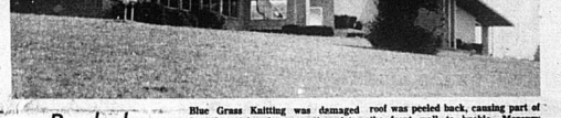
Blue Grass Knitting was damaged roof was peeled back, causing part of Saturday night when a portion of its front wall to buckle.—Mercury
