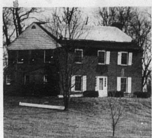
A severe wind and hail storm broke in Nicholas county Wednesday afternoon, April 2, between 4 and 4:30 p.m., causing the damage shown to the home of Mr. and Mrs. Nate Young, Paris Road. The porch roof was blown on top
