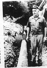
Hervey E. (Pete) Gaunce, farm manager for Ashby farm helping put pipe through end of pond fill to carry excess water.
