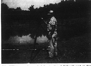
Otis Williams, employee of Soil Conservation Service, overlooking construction of McDonald pond on East Union Road.
