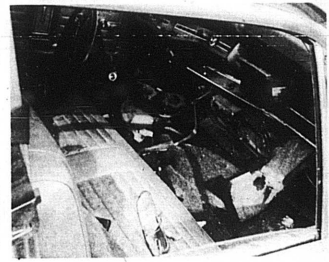
Column can be seen the buckled steel of the fire-wreck. See story elsewhere—Mercury picture.
