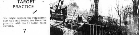
2 Another View Looking up stream at the underside of both truck and bridge as workmen peered to right truck with the aid of cables, pulleys and wreckers.
