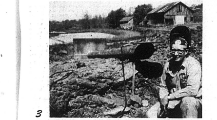
CRAIG BARTON installed two anti-sweep collars and a hood on an eight inch mechanical spilly on the Rogers farm. Anti-sweep collars prevent water from following the pipe. The hood is an anti-vortex device that prevents the water from swirling like sometimes seen in a sink or bathtub, thereby making the pipe more efficient by carrying a full load.
