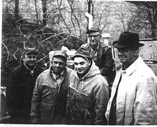
Charles Whaley, right, representing the Nicholas County Soil Conservation District Board of Supervisors, was present when the new bulldozer, recently delivered to Mike Tucker, (center), and Paul Gaultier, (left), started work on the farm of Grover Livingston, extreme left.
