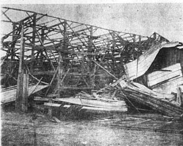
COMPLETE LOSS—High wind last Wednesday night, Feb. 15, played havoc with this barn, the property of Berry Wilson. The 84' x 64' structure is located in Bath County.
