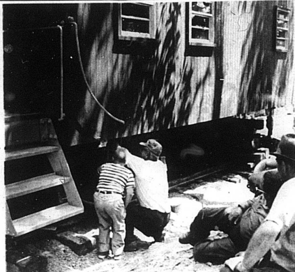
THESE CLAMPS WORK!—Special bolts and clamps were put on the engine springs to lift the trucks up enough to keep them from touching.
