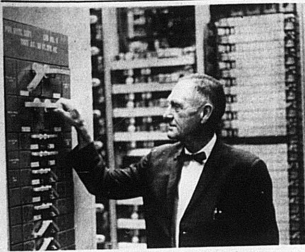
SWITCH THROWN—COUNTY JUDGE FLOYD CLARK IS SHOWN AS HE PREPARES TO THROW THE CIRCUIT CONTROL IN THE PRESENT DIRECT DISTANCE DIALING CONVERSION AT CARLISLE.
