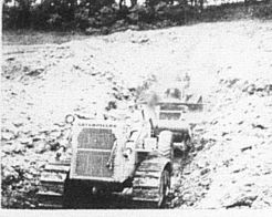
EARTH MOVING—Doug Norman and Ted Hunter, operating some of Fred Jones' heavy equipment, are constructing a big pond on the Norwood and Dean Jansen farm. This is one of the first conservation "contract" jobs undertaken in the county. Farmers, like other businessmen, like to know in advance the cost of applying planned conservation practices before construction. Especially is this true for big projects costing several thousands of dollars. Usually earth moving work is done at an hourly rate. To enable the farmer to know the exact cost of a specific practice, Fred Jones has started contracting to do specified practices to meet plans and specifications prepared by the Soil Conservation Service.
