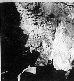
WHAT A HOLE, MANHOLE, THAT IS!—Seventeen feet through solid rock to Ernest Sosby says. He's the fellow who took the picture at the location of the new County nursing home on the county farm west of Carlisle.
