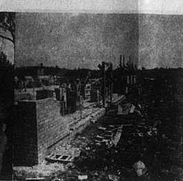
CONSTRUCTION PROGRESSES—At left part of a sewage disposal plant. Right, the Nicholas County Home, abiding.—Photos by Ernest Sosby
