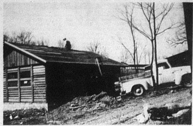
Work is progressing on the District 4-H Camp. In the above picture, Harry Trapp, camp director, sits atop the 2000 cubic container on the site. In the far background can be seen the shelter house which will be used for handicraft, meetings, and other activities when it rains. Plans are completed for the kitchen which will be one of the finest of any camping facility anywhere in the U. S., reports John Perkins, chairman of the camp planning group. If you have not visited the camp, drive out and look around — you'll see for yourself just what has been done. Plans are to start camping at the camp in 1966.
