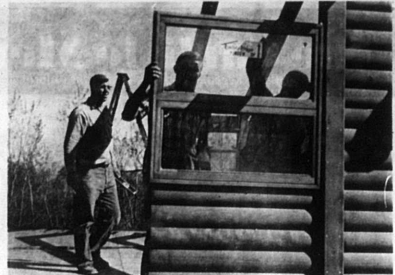
CONSTRUCTION OF A TIMBER-LODGE—Shown above are some of the construction on steps in reaching the well-crooked home. Top pic Ed Cox and Harry Trapp in window into place. Middle pic, roof begins to take shape, erection time thus far only one-half day, Bottom, raising a frame into place, Cox and Trapp again. Carlisle, Ky. home was finished in four and one-half days.
