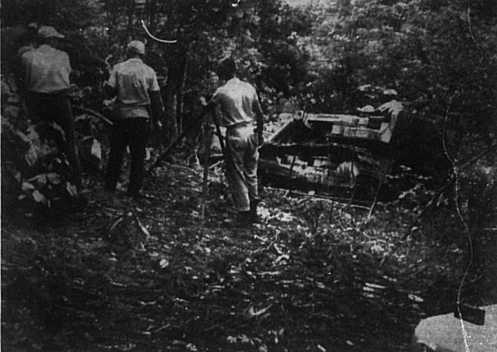
ALL WILDERNESS —Plenty of trees and evenly pollinated camp sites abound around the Nicholas County Lake. 2 1/2 miles northwest of Carlisle. State Highway Engineer Tom Price of Georgetown, center, adjusts his transit while Billy Brown, donor operator clears the underbrush for the survey crew. At extreme left, Clifton Waugh, Caterpillar owner helps cut down Stanley Alexander, another Miles an employee of Dorsey Watkins looks at the thicker head and wonders how many staks he'll have to drive before the job is finished. In the lower right corner "Old Bertha" Mr. Watt
